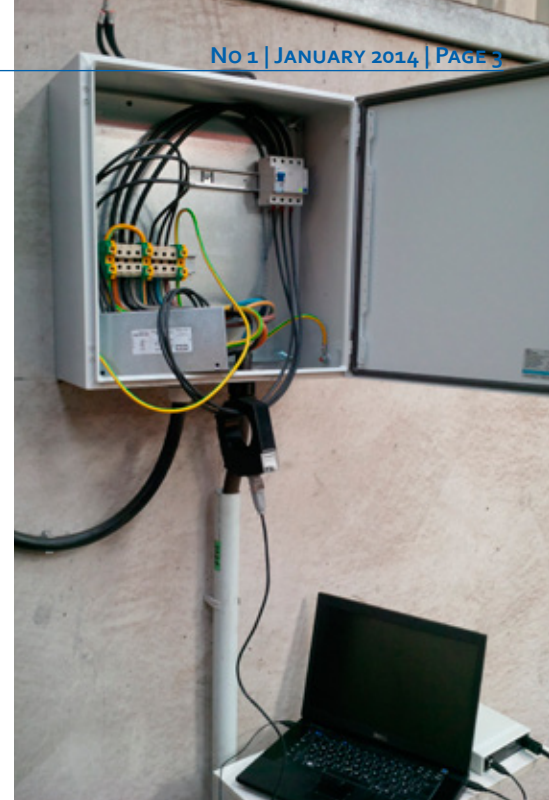
▲ The test set-up: DRCA 1 and notebook in the bottom right of picture. The converter is only fitted loosely for diagnostics. The loosely installed EMC filter, fitted for test purposes, is in the bottom left of the distribution box.
